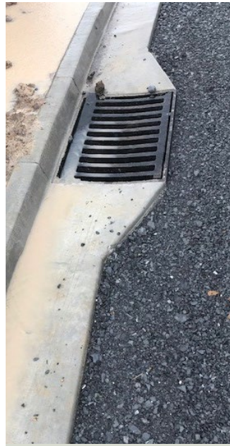
Figure 1: Sediment discharge due to inadequate stabilisation of site entranceway.
