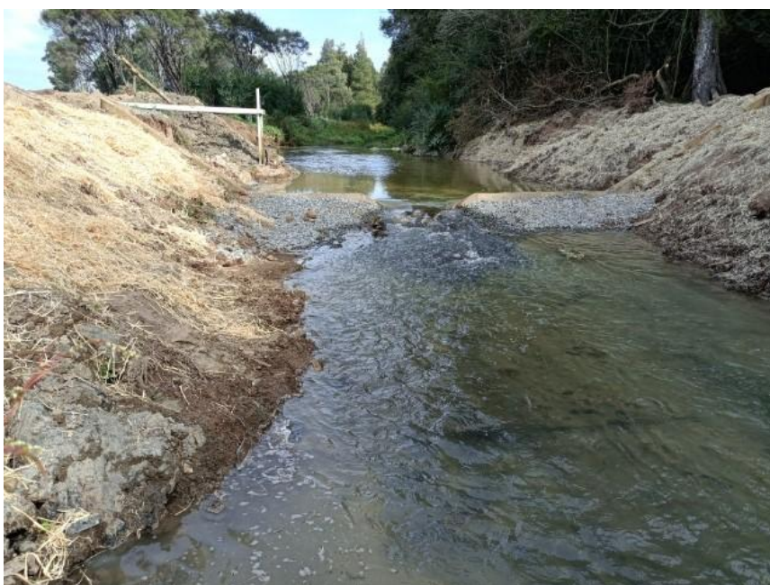
Figure 20 Flow monitoring weir on the Waitoa River at Waharoa. This photo was taken May 2022 after the weir was rebuilt (photograph Kane Lynn).
